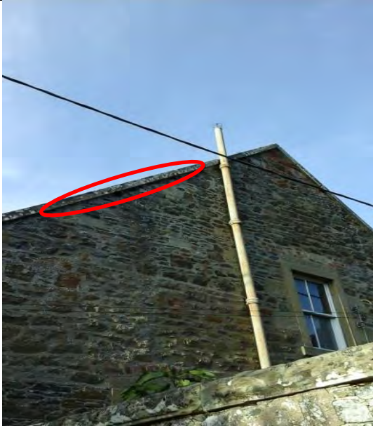
Building with High BRP. Gaps under roof
